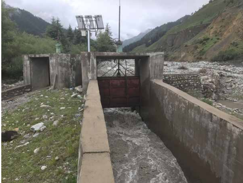
Fig. 19 Channels with Shallow Water and Washed-away Rocks
